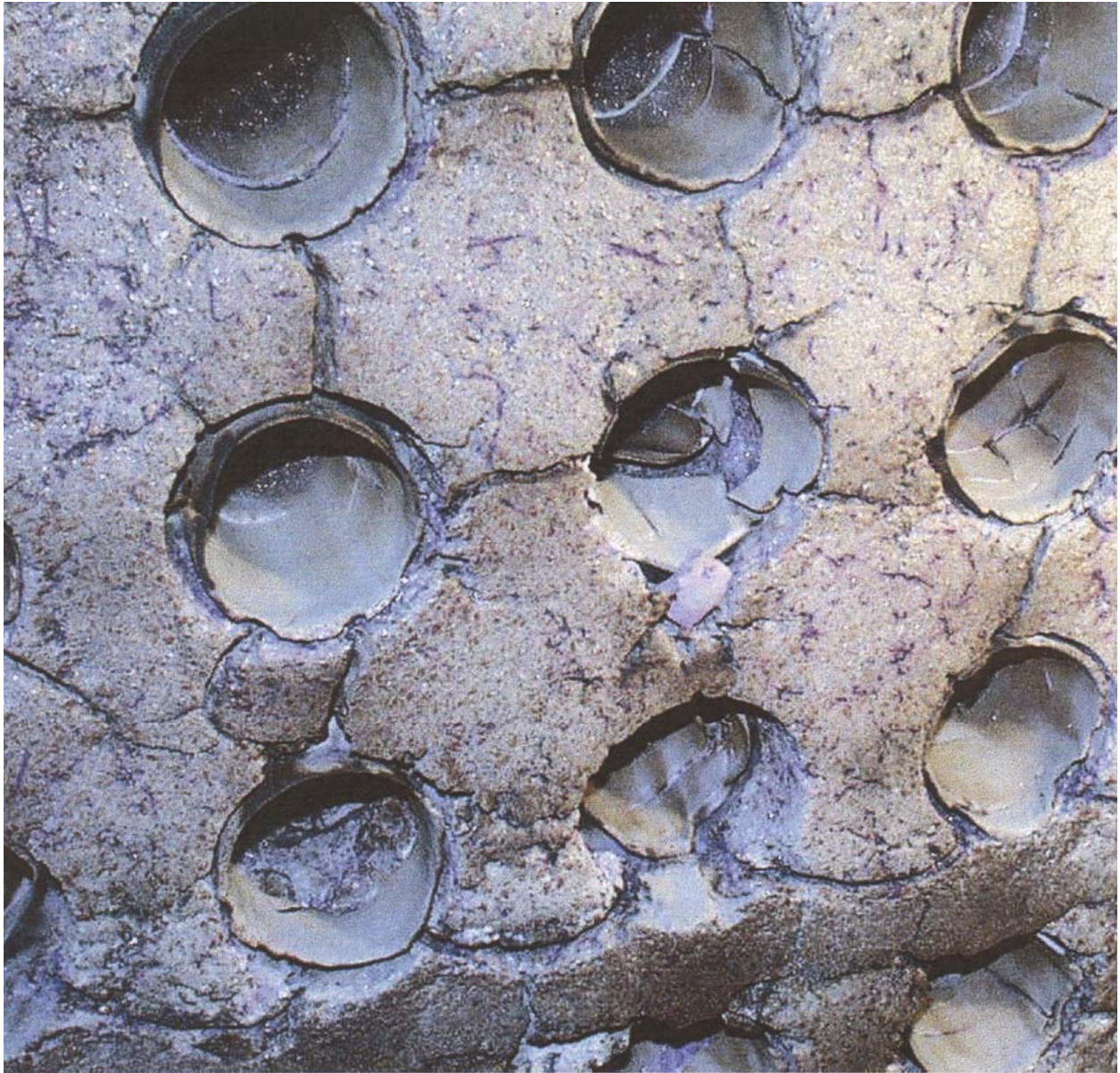
Refractory Damage from Wrong Material of Construction
